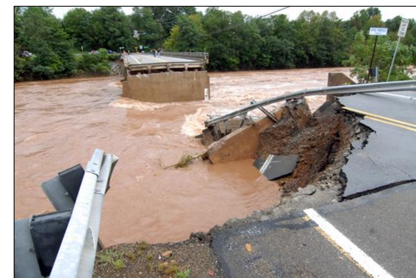
Figure 6. Flooding on Loyalsock Creek destroyed the bridge over Rt. 973 in Loyalsockville, PA. The USGS stream gage at this site was disabled due to the record high flow. (Photo: PA State Police)
