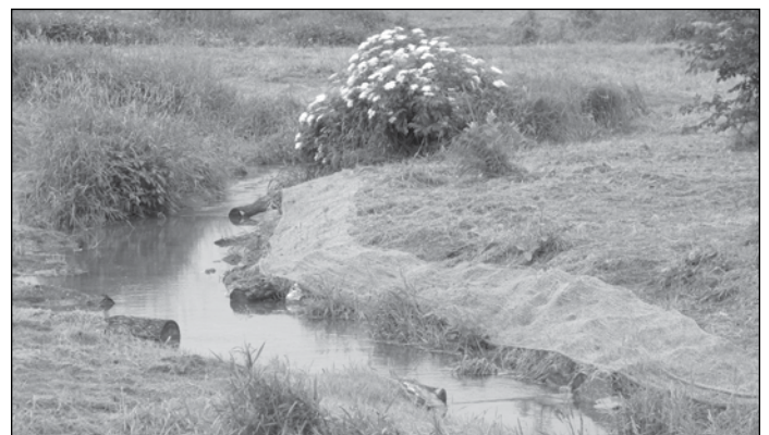
Several landowners along Limestone Run in Montour County have partnered with PA DEP, PA Fish and Boat, the Montour County Conservation District, and Northcentral Pennsylvania Conservancy to install multilog vanes and muddills to stabilize the stream banks, eliminate eroding stream banks, and create fish habitat.
